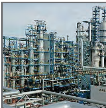
TAIF-NK VCC LLE2 PROJECT (Tatarstan - Russia) (Ignition System for Burners - 2014)
